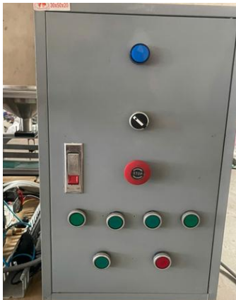
a) Exterior view of the control cabinet
