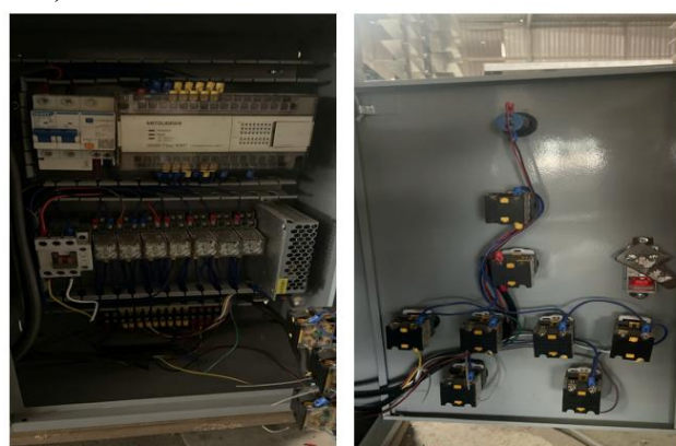
b) Internal view of the control cabinet
