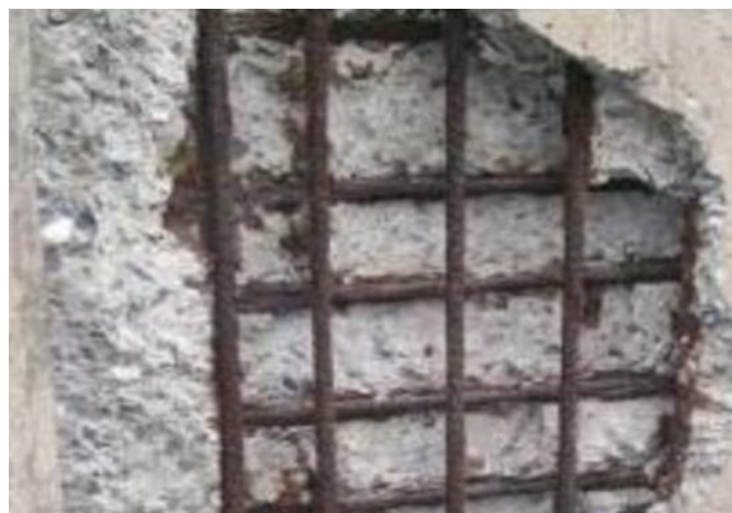
Figure 2. Steel corroded despite the protection of concrete
