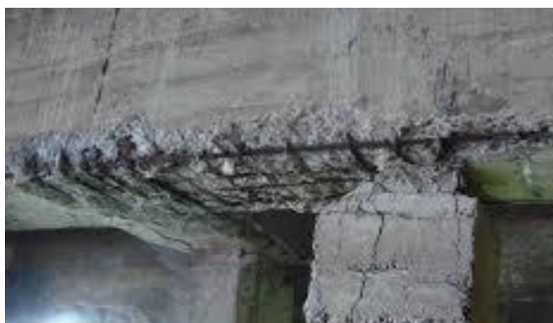
Figure 1. Corrosion of reinforced concrete beams
